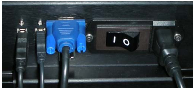
Figure 7-2: Main power cable and switch
