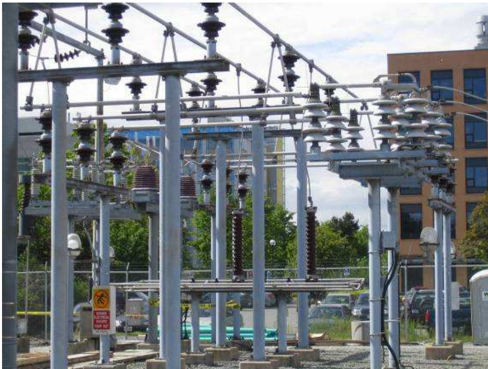
Figure 4.5: UBC Substation feeding power to whole campus
